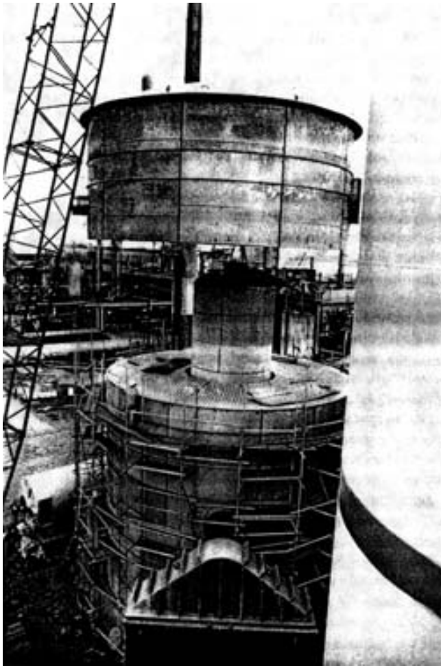
Last stage of assembly of the first all-austenitic, nickel stainless steel converter for a 1200 ton-per-day, energy efficient sulfuric acid plant. Note the heat exchanger within the converter in this proprietary design.
